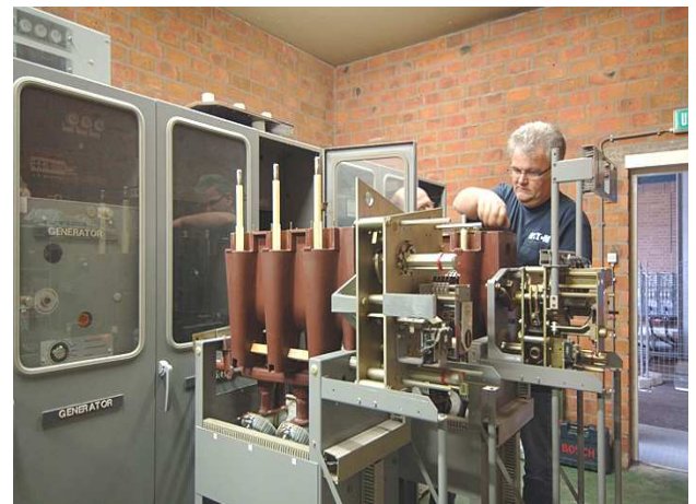
Fig.1 Maintenance of 30 years old minimum-oil breaker.
