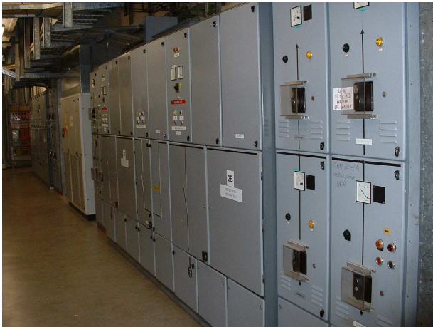
Fig.4 Current switchgear configuration
